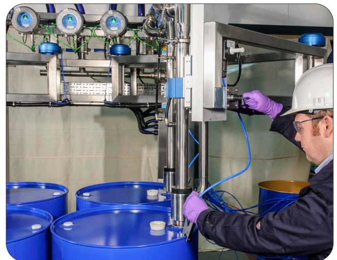
Fig. 2: Pulsing green ground status indicators provide operators with a visual reference point to ensure the equipment they are operating is grounded prior to, and during, the operation.
