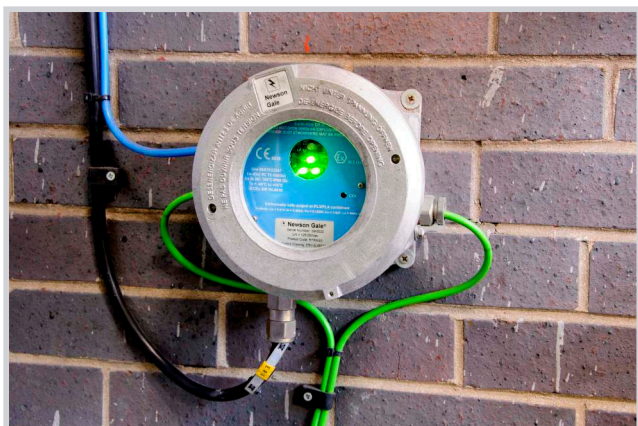
Figure 2: Traditional wall mounted ground status indicator system with internal output contacts. Note the green for 'SAFE TO GO' indication method.
