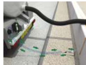
Continuous Ground Loop Monitoring check
